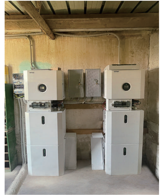
09 Residential ESS Project in Italy
