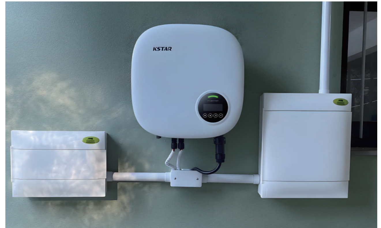
11 Residential Solar Project in Brazil
