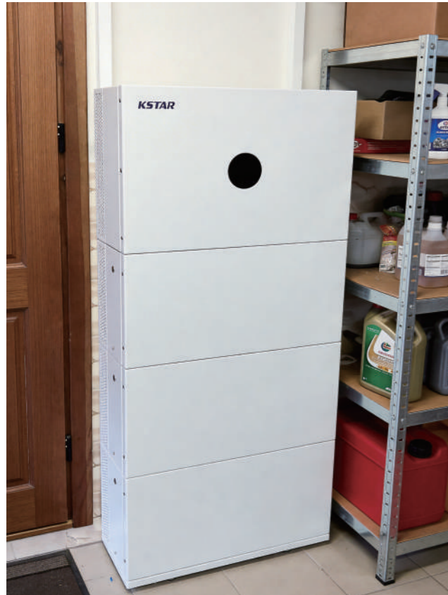
01 Residential ESS Project in Lithuania
