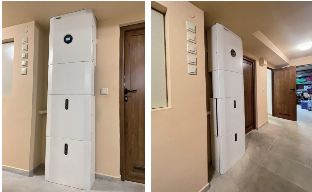
07 Residential ESS Project in Bulgaria
