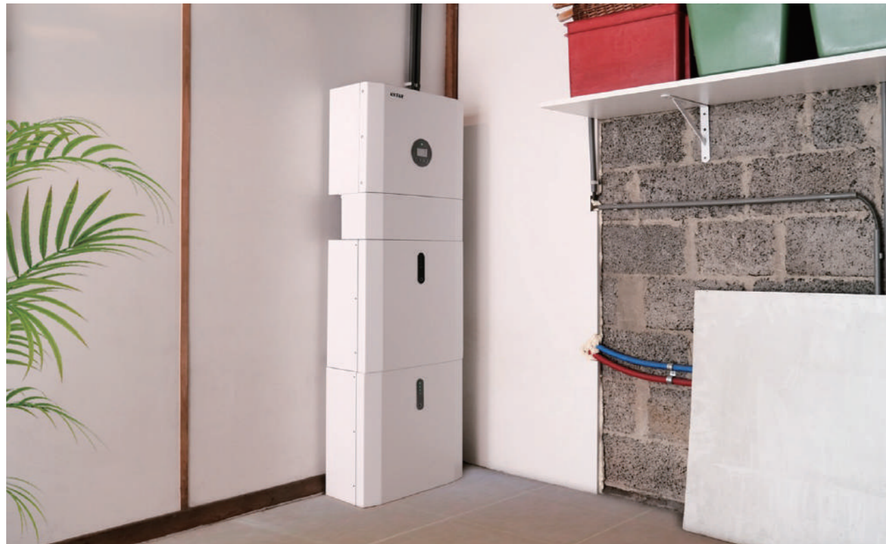
10 Residential ESS Project in the Netherlands
