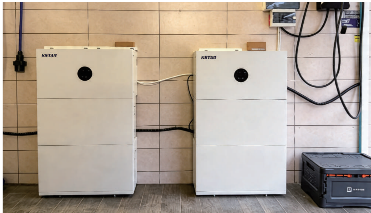
05 Residential ESS Project in Ukraine
