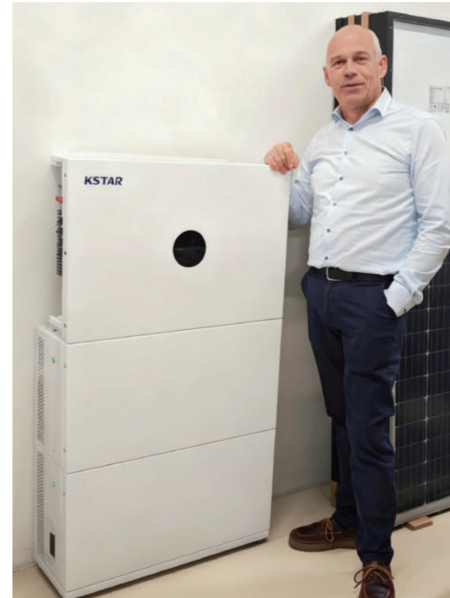
03 Residential ESS Project in the Netherlands
