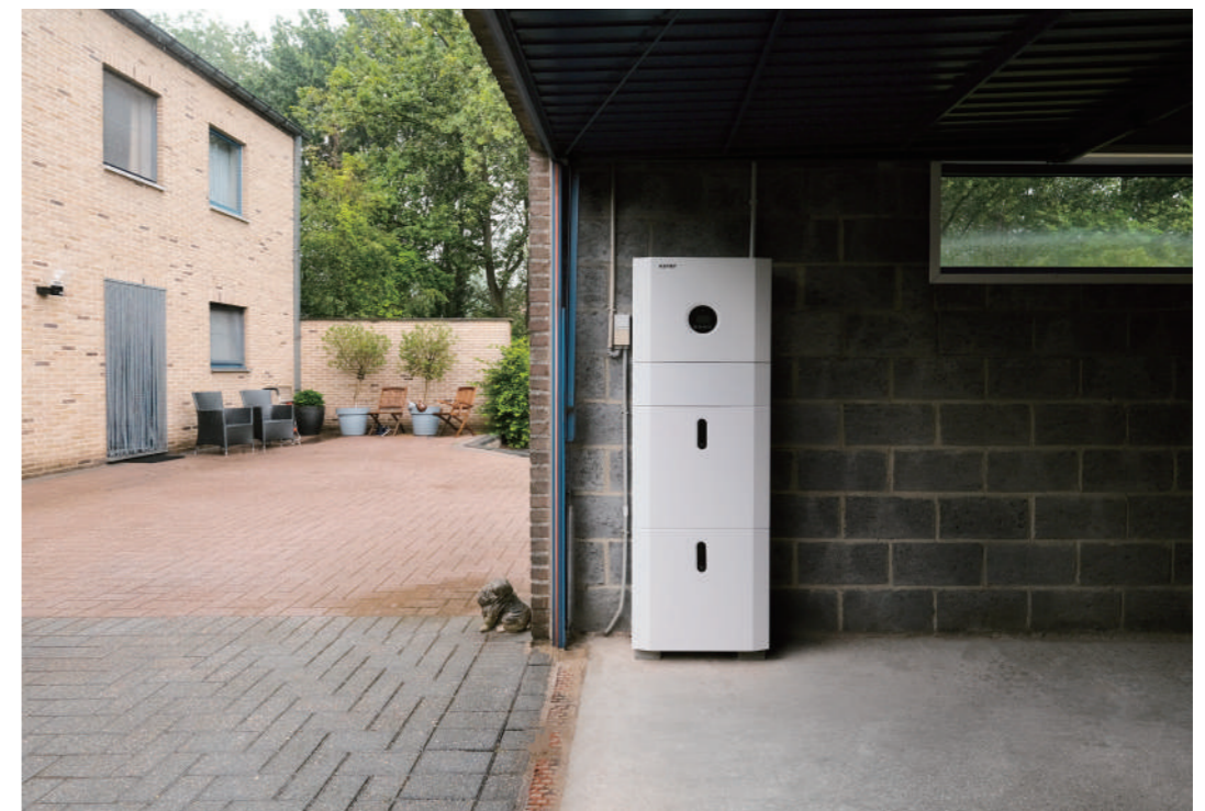
15 Residential ESS Project in Belgium
