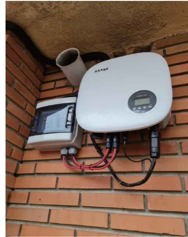
08 Residential Solar Project in Brazil
