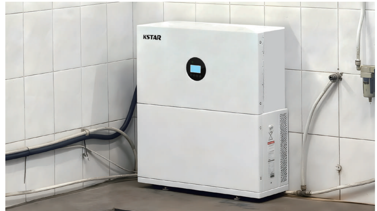
06 Residential ESS Project in Ukraine
