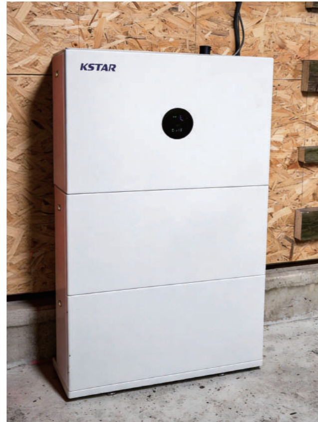
02 Residential ESS Project in the Netherlands
