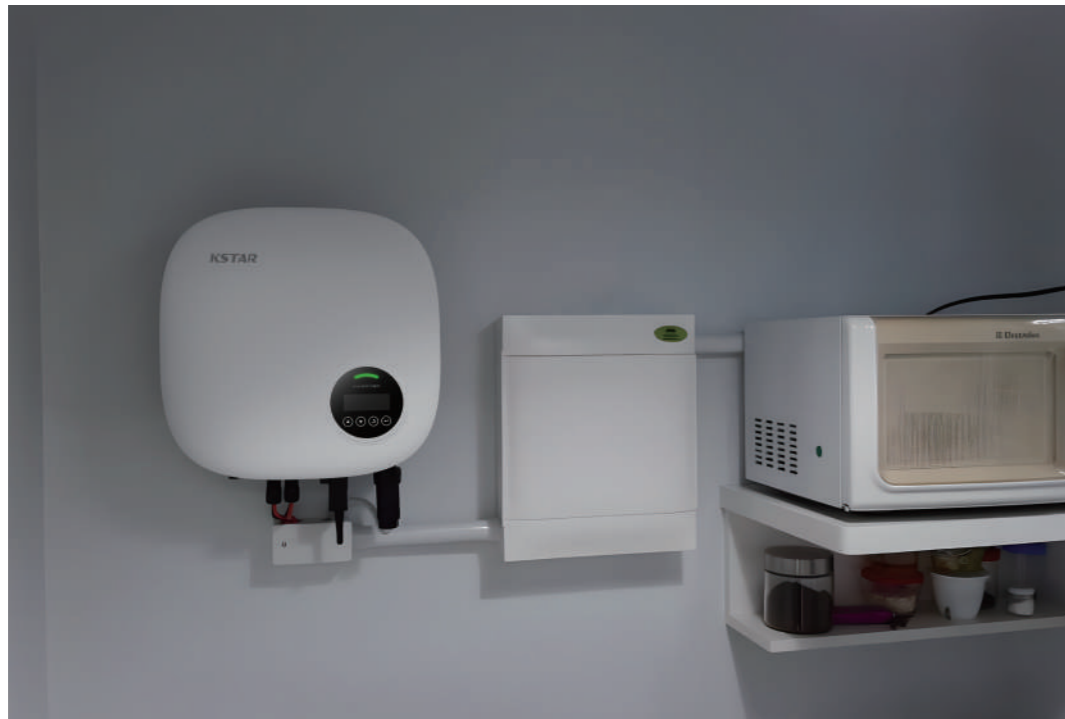
14 Residential Solar Project in Brazil
